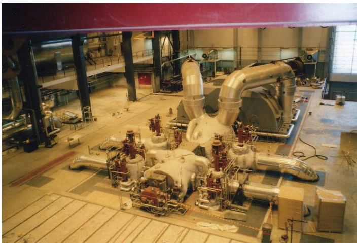
Figure 5: Alholmens Kraft Turbine Hall Showing 240 MW Steam Turbo-Generator
