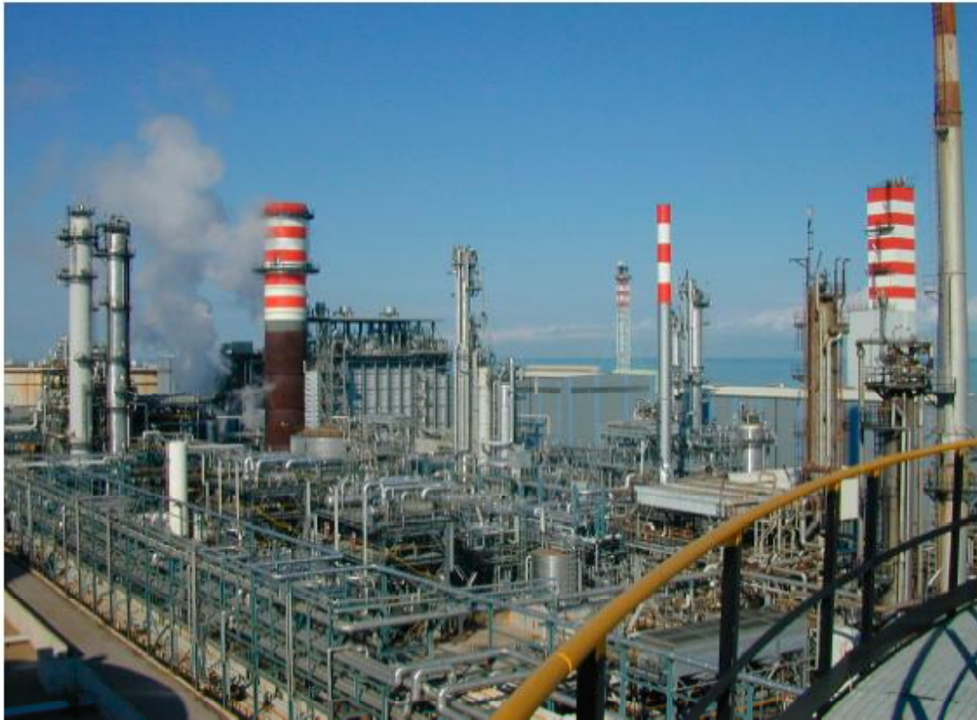
API Falconara IGCC, 290 MW Cogeneneration with ALSTOM 190 MW GT13E2
